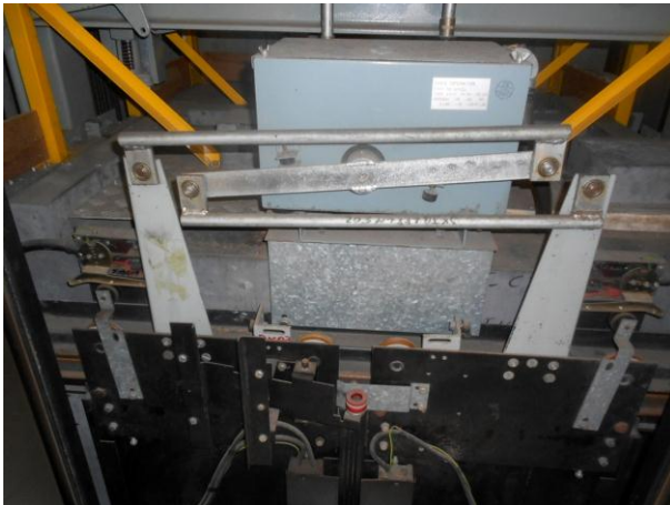
Photograph No. 3 – Car power door operator
