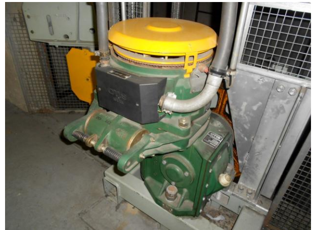
Photograph No. 2 – Geared lift machine
