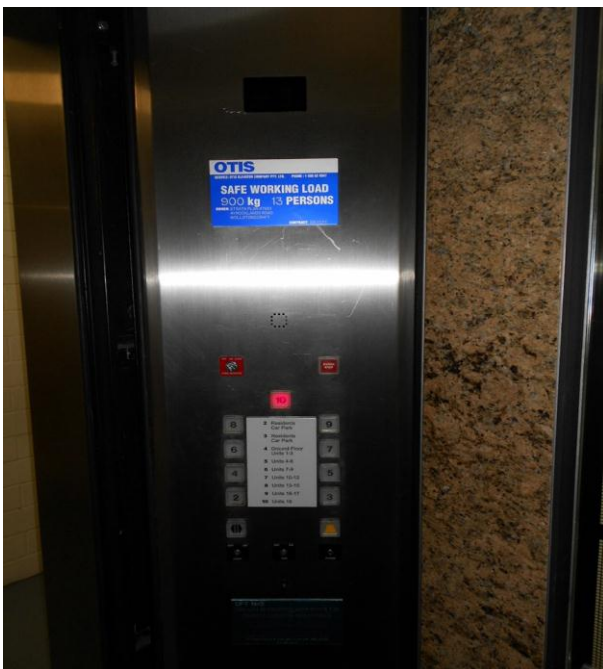
Photograph No.5 – Front splayed car operating panel
